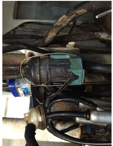
Pulsator line and cracked inflations
