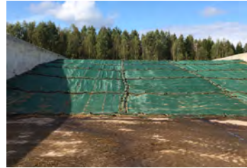
Better approach: gravel bags create a good barrier against air penetration under the plastic. Bird net prevents cover against damages by birds.
